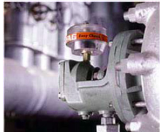
Figure 2: Entry level monitoring device installed on a pump
